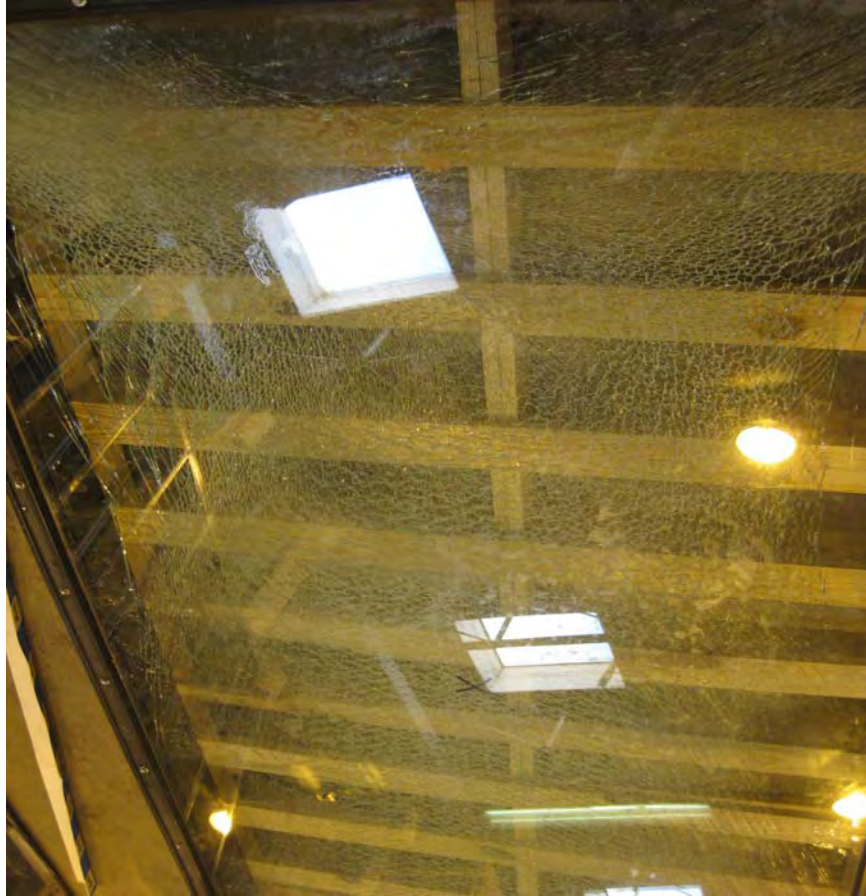
Photo No. 2 Laminated Glass Fracture at 7' Drop
